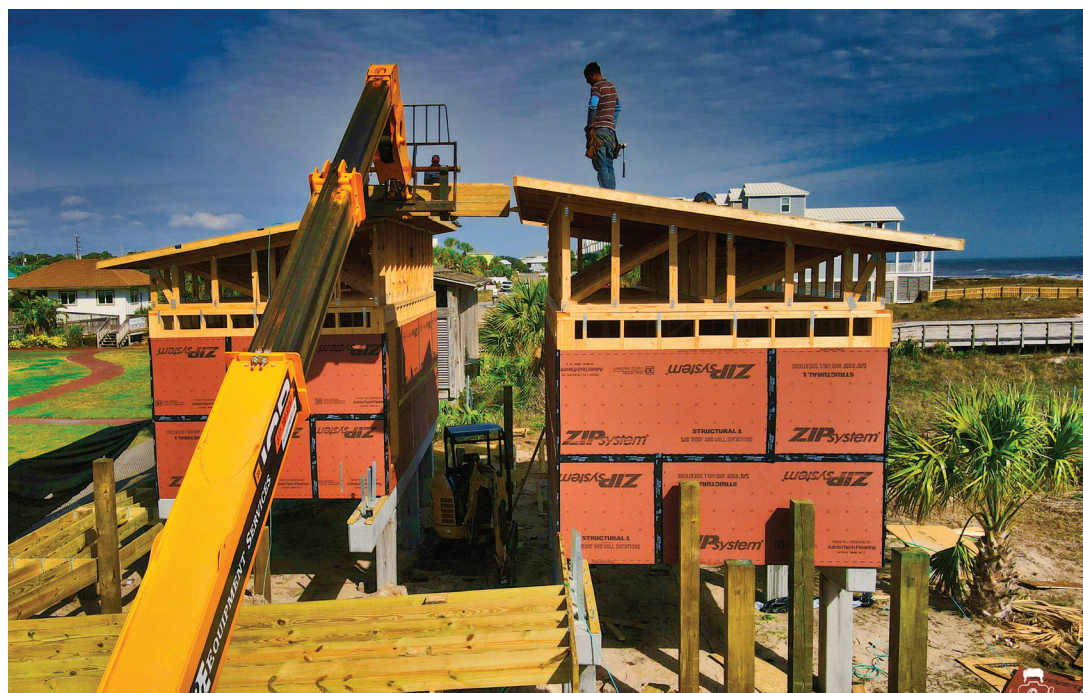
Restrooms taking shape at Lighthouse Park show the separate women’s and men’s areas. Photo by Michael Yelvington
