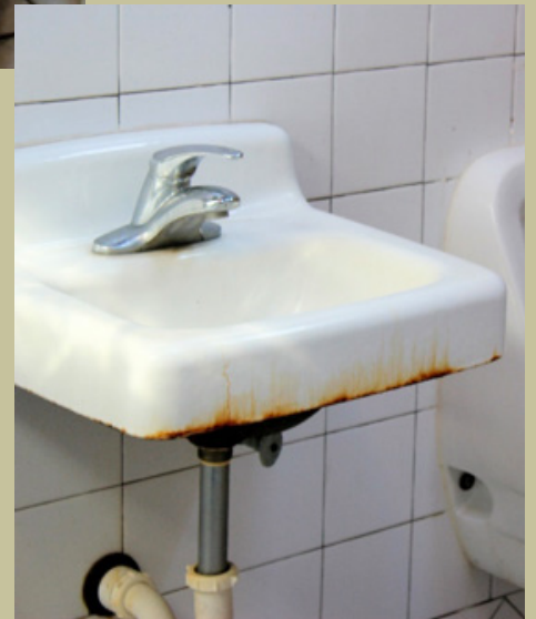
The facilities at Lighthouse park are not handicap accessible and are grossly inadequate for the 50,000 visitors who come here each year.
